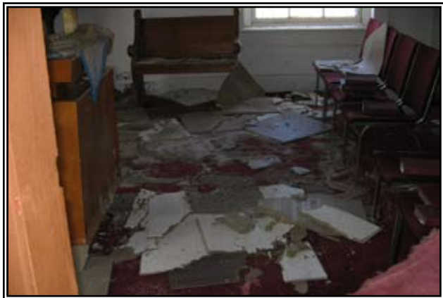
What was once a chapel, with ceiling parts on the floor
