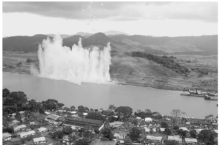
Work on the expansion to the Panama Canal started with a spectacular explosion.
